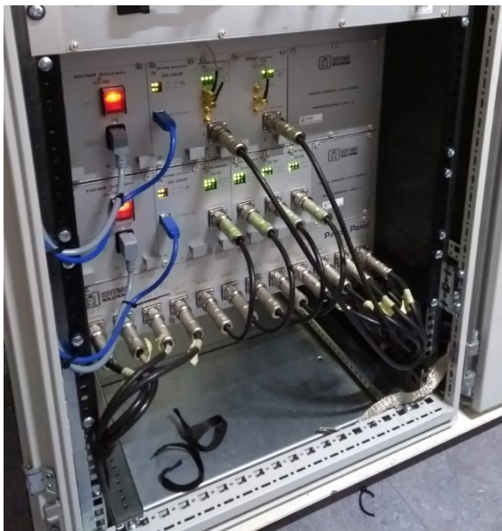
Figure 7: ERTMS Solutions TLC On-board rack
